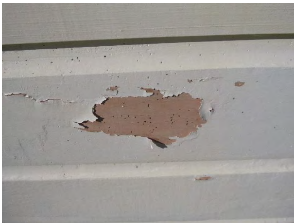
Photo 9: Paint flaking off the timber cladding on the dwelling.
