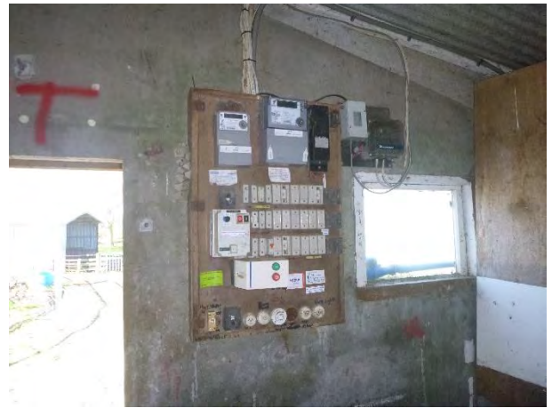
Photo 20: Fuse box situated on the inside wall of the milking shed.
