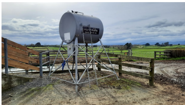
Photo 9: Above Ground Diesel Tank
