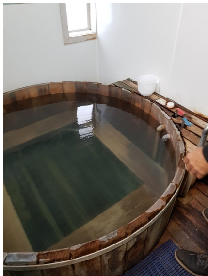
▲ Plate 2.3: Deteriorating spa finishes.
