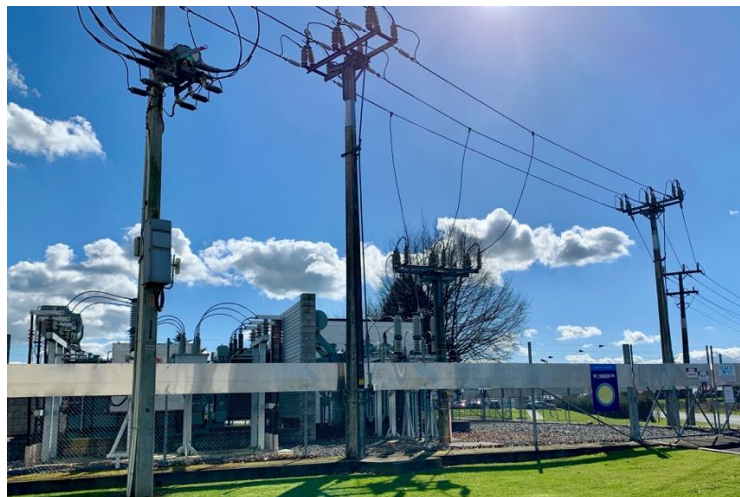
Figure 5: Waharoa Electricity Substation
